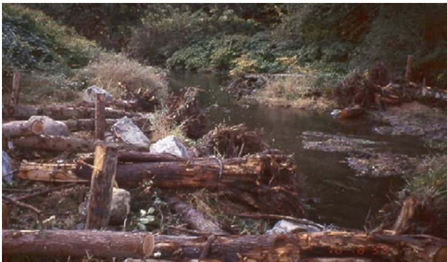
Plate 5 LWD dam anchored using a combination of rock ballast, cabling and pilings (Stream Habitat Restoration Guidelines (2004)).
